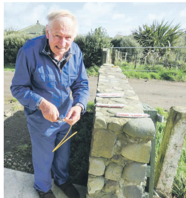
Len Pentelow with the equipment used to lay explosives. Of the inspectors he says they're more interested in you not blowing up other people.
